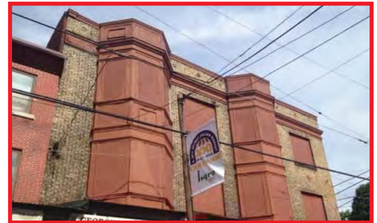
It is not recommended to board up or close upper story windows in any fashion.
