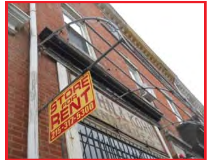
Retaining the metal armature of an awning attached to a building without its canvas covering is not recommended.
