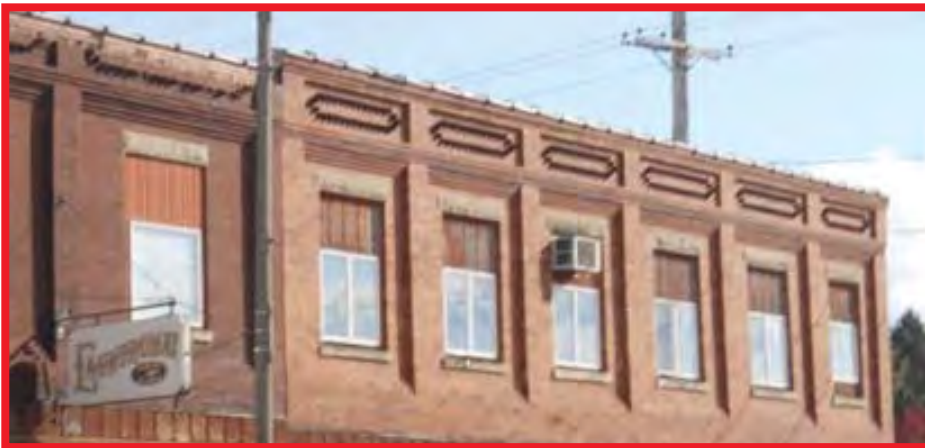
It is not recommended to reduce the window size to an area smaller than the original, as seen here.
