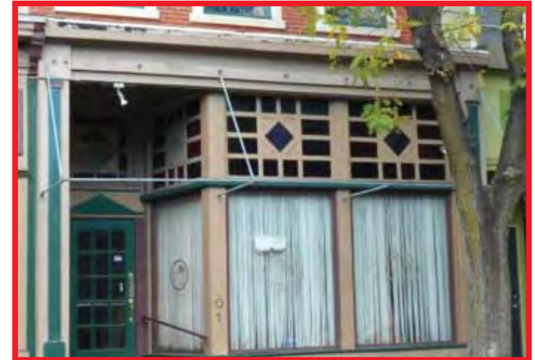
Covering architectural details, such as these transom windows, with continuous awnings or oversized awnings is not recommended.
