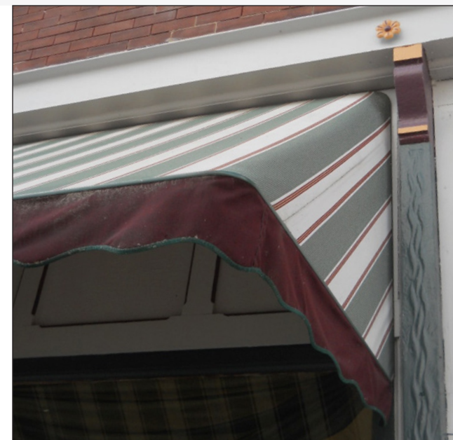
This handsome striped canvas fixed awning is placed within the cast iron frames of this storefront in Moline IL. The colors for the awning and valance match the colors of the building itself.
