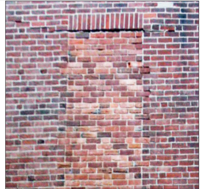
Filling in upper story windows as shown here on a building in Gloucester City NJ, creating windowless blank walls, or destroying original architectural details is not recommended.
