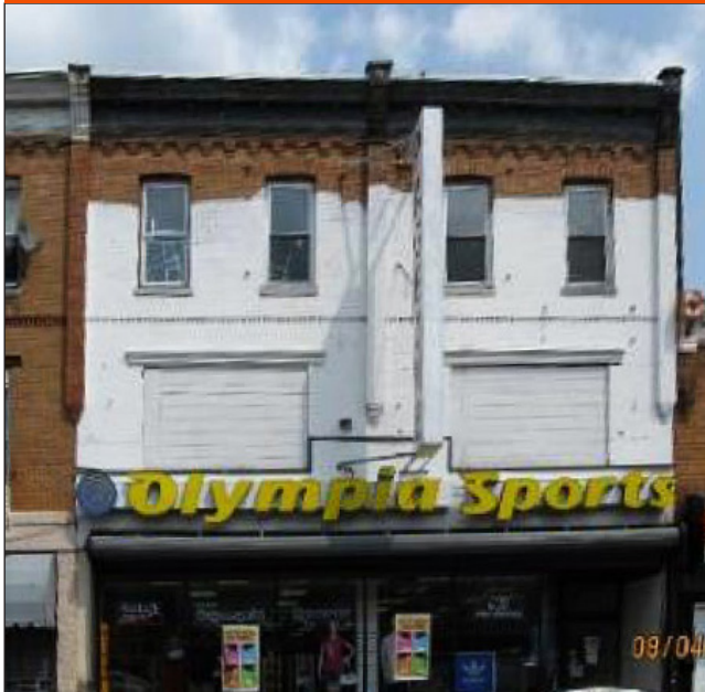
It is not recommended to paint brick (see above), stone, tile, stucco, or molded concrete block if they have never been painted before, as seen on this building in Philadelphia. The unpainted elements have a natural or man-made finish that is important to preserve.
