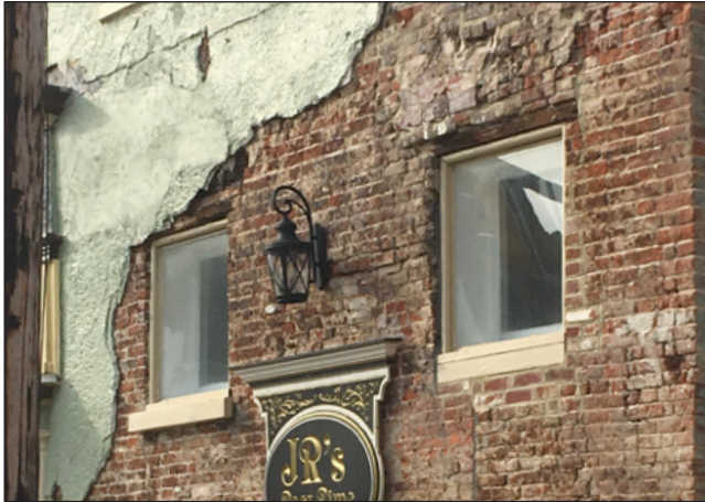
This wall was once stuccoed over, and has not been repointed, leaving a scarred and poorly maintained building in the heart of downtown Smyrna DE.
