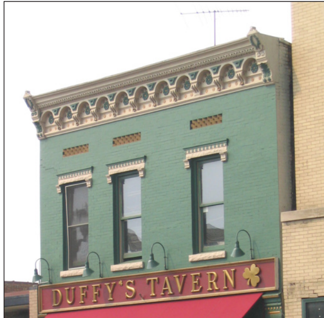
Masonry buildings that are already painted, like this one in Forest Park IL, should continue to be painted. This building and storefront have been painted in harmonious colors that highlight the important historic features of the building including the wood cornice, upper story window frames, window hoods and window sill.
