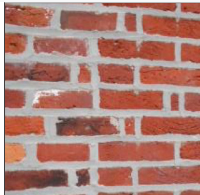
The surface of the brick seen here on a Philadelphia building has been eroded by sandblasting in the past. Sandblasting is not recommended for any masonry or brick building in Seaford.
