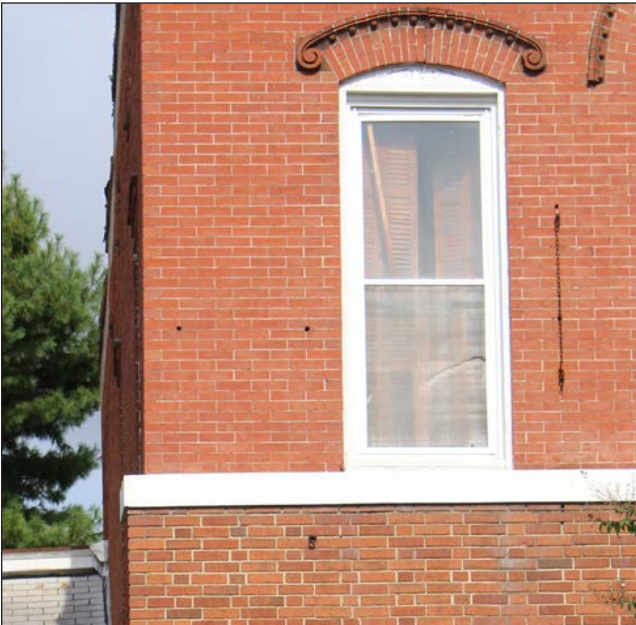
Note the different brick patterns at 312 HighStreet. The original brick is laid in a common bond brick pattern with a very thin mortar joint above, often called a butter knife joint. The brick installed later, below the white stone string course, has a slightly different color, and is laid in a Flemish bond brick pattern with slightly wider mortar joint.
