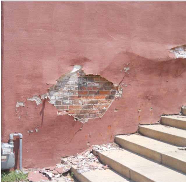
Poor maintenance practices can lead to more significant and expensive problems in the future. At some point in the past, this wall in Moline Illinois was stuccoed. Moisture has seeped into the wall, causing the stucco to pop off, presenting this unattractive wall to the public. Not addressing wall problems like this only lead to more expensive repairs later.
