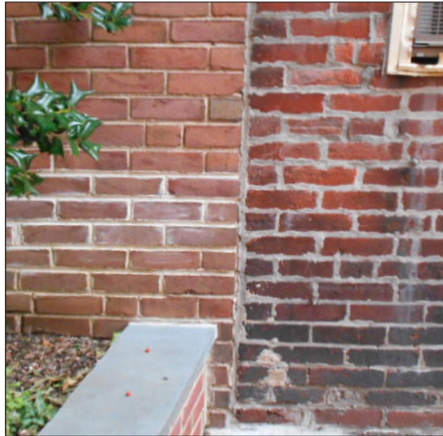
The pointing in the upper left-hand portion of this brick building in Philadelphia has been pointed correctly, while the brick pointing on the right side has been poorly applied. The right side shows where the new mortar has been permitted to "feather edge" onto the face of the adjacent bricks, which is not recommended.
