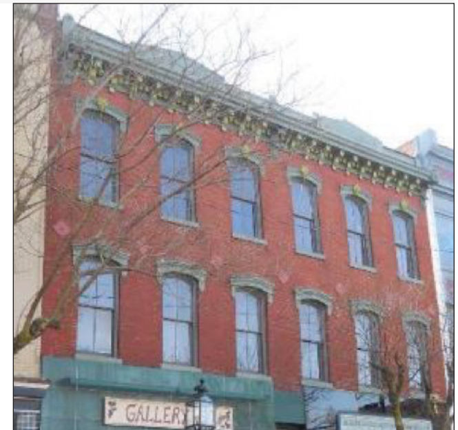
The two over two light replacement wood upper story windows for this building in Bridgeton New Jersey fill the entire window opening.
