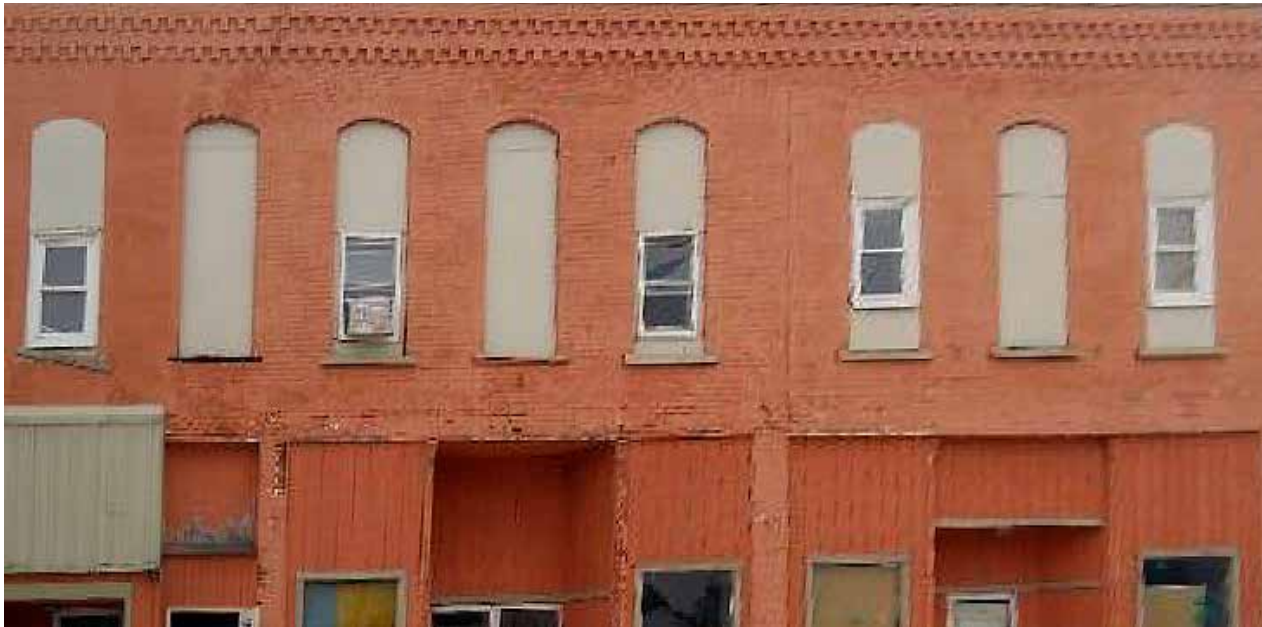
It is not recommended to board up or close any upper story windows in any fashion, as seen here on a building in Aledo IL.
