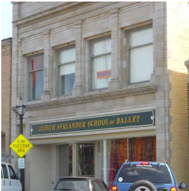
It is not recommended to reduce any upper story window size to an area smaller than the original, as seen here on a building in Aledo IL.
