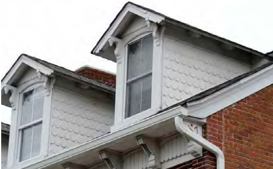
Milford's downtown is fortunate that it retains a great deal of its original historic buildings. The Windsor Building at 24 NW Front Street, home of the Greater Milford Chamber of Commerce, retains the handsome shaped shingles on the dormer windows, along with carved brackets that hold up the gable roof. This Italianate style building also has its original wooden bracketed cornice.
