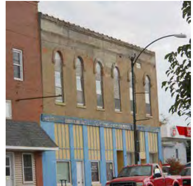
It is not recommended to reduce any upper story window size to an area smaller than the original, as seen here on a building in Aledo IL.
