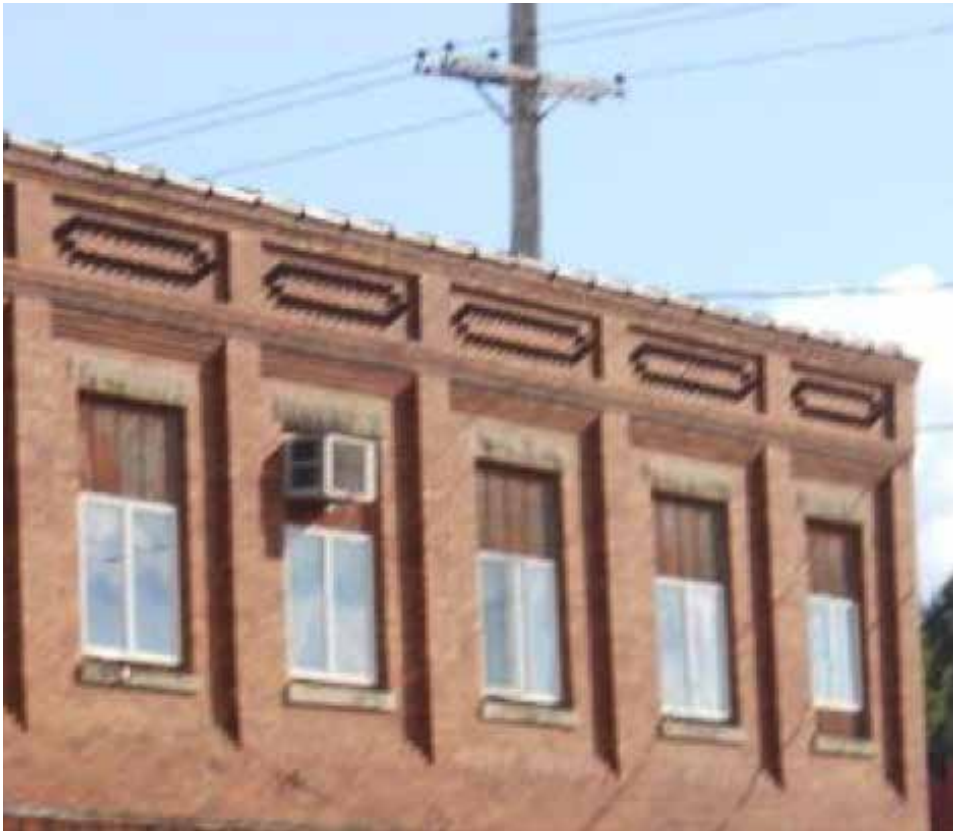
It is not recommended to reduce the window size to an area smaller than the original, as seen here on a building in Prophetstown, IL.
