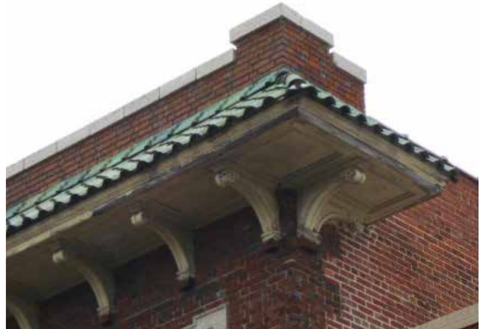
Retain any historic cornice like this one at 124-126 East Market Street. This cornice is made of wood with handsome wood brackets that hold up the green terra cotta roof tiles. Keep any original upper story masonry, wood, and metal cornice intact. Decorative cornices in Laurel are important to preserve. If they are deteriorated, they should be repaired rather than removed.
