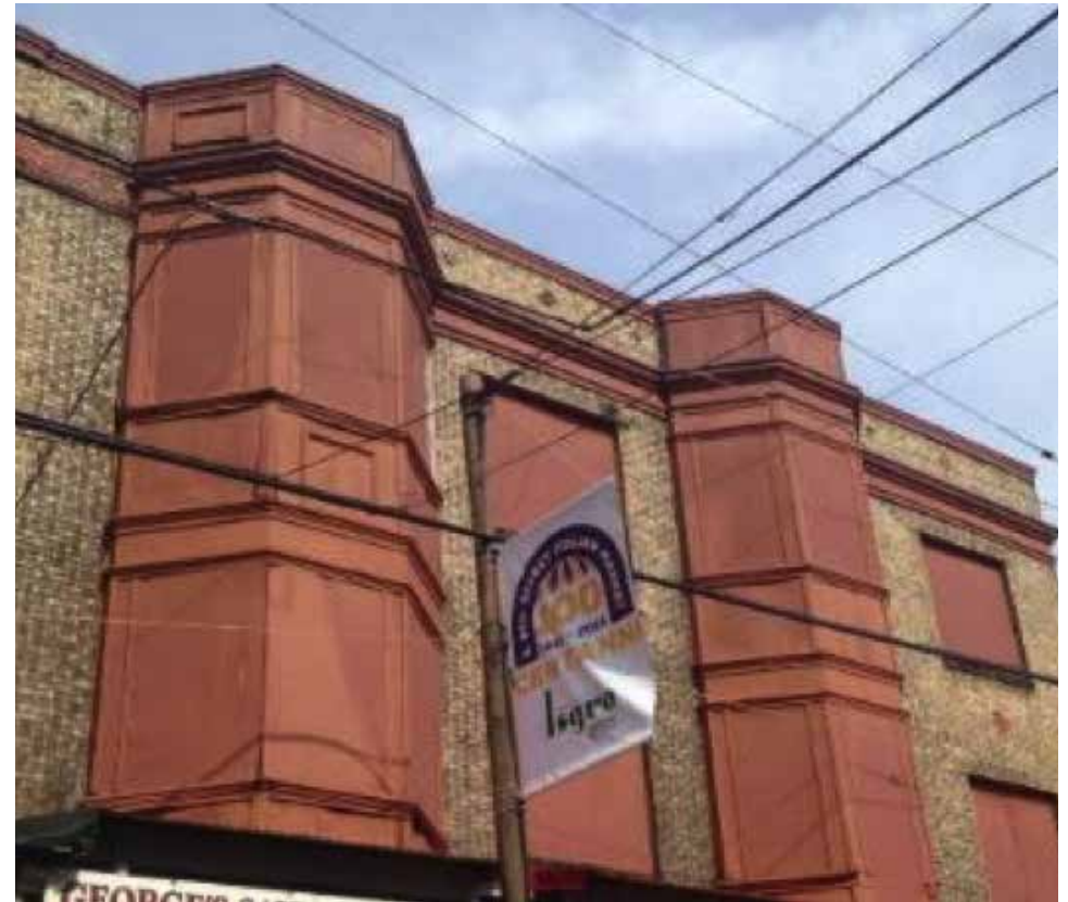
It is not recommended to board up or close upper story windows in any fashion, as can be seen here on a Philadelphia commercial building.
