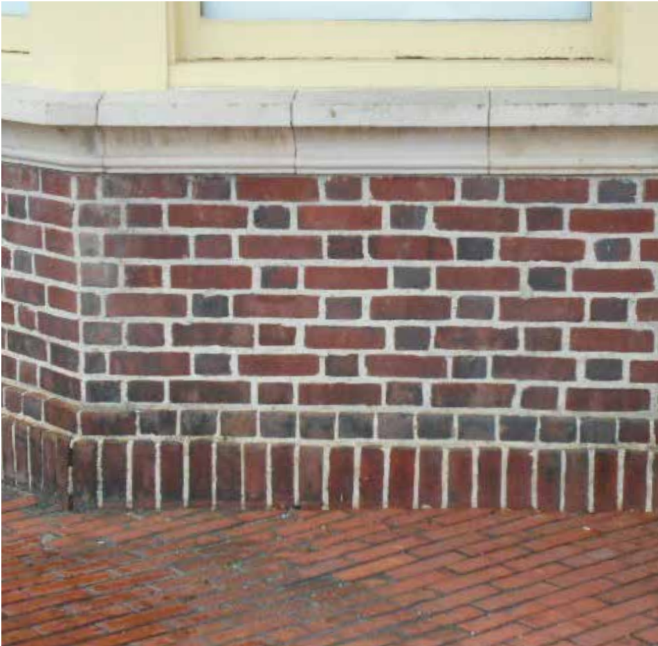
Repointing of the historic train station on Mechanic Street was done with great care to match the mortar color and texture and to ensure that the tooling matched the original.
