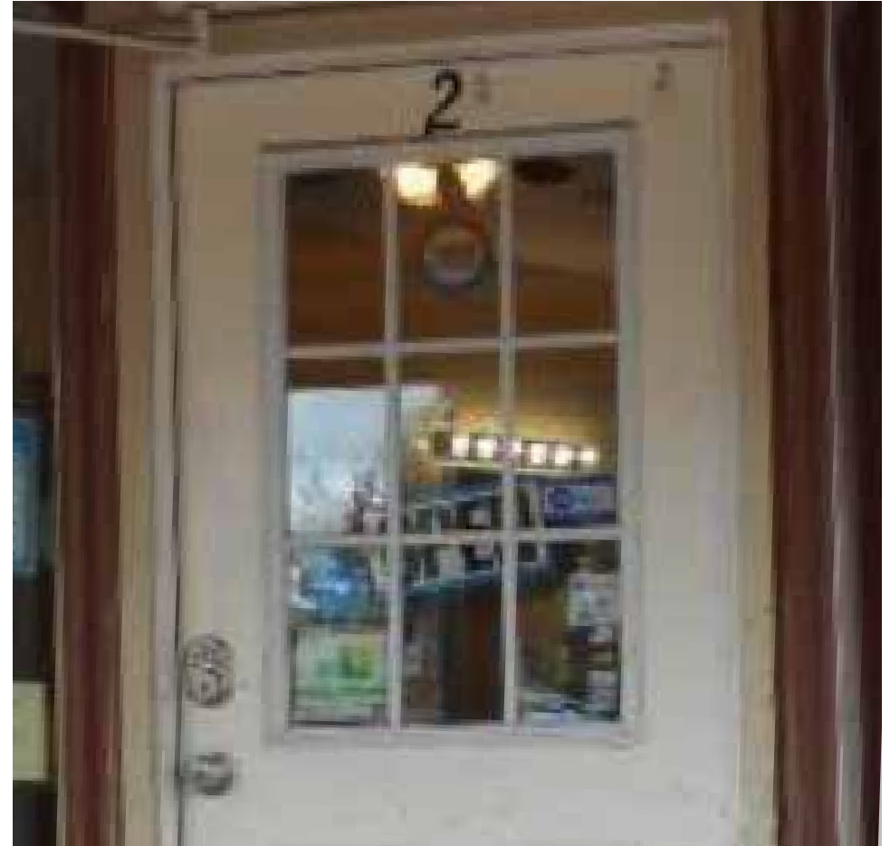
It is not recommended to use doors that are more suited to residential use for commercial entrances like this one shown here from West Orange, NJ.
