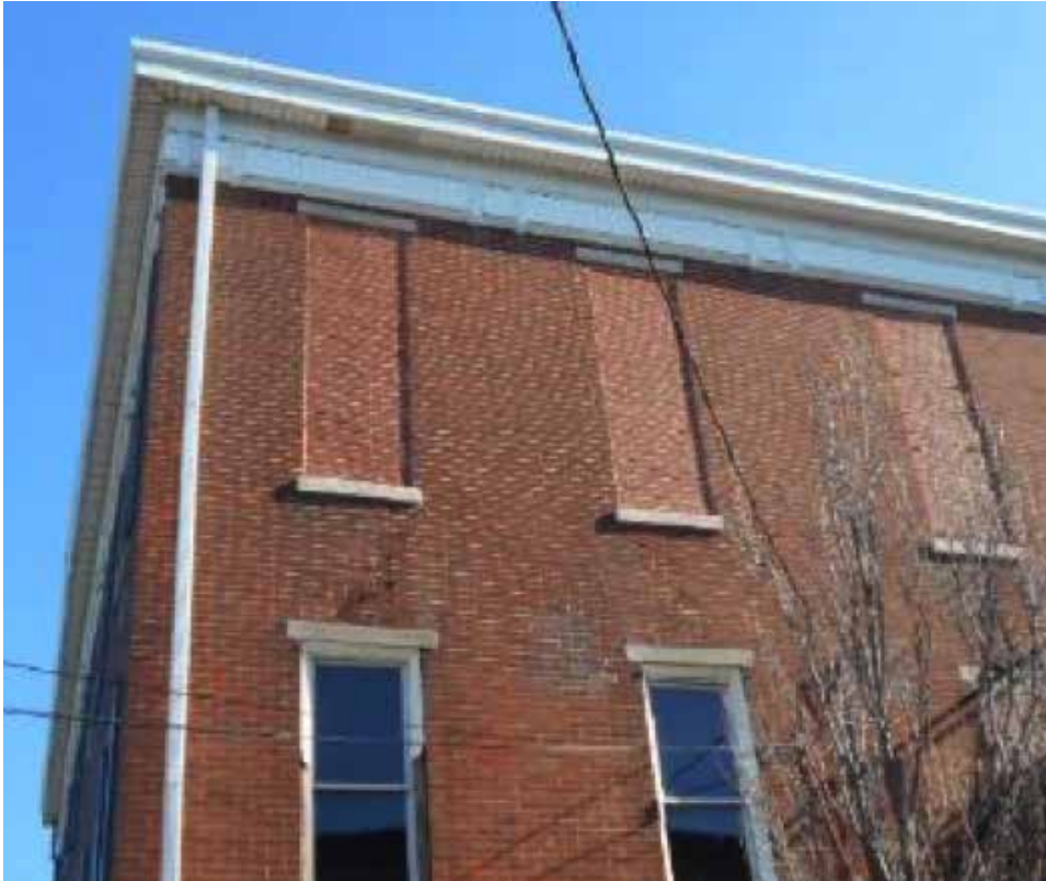
Filling in existing window openings, as seen here on a building in Gloucester City NJ, is not recommended on upper facades.
