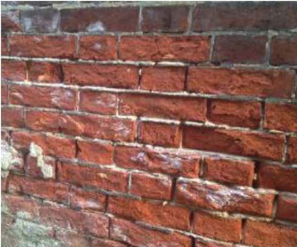
Sandblasting (see results above) and cleaning with harsh chemicals are harmful to masonry and brick when used to remove paint or dirt from any masonry surface and are not permitted in downtown Laurel. Photo from a building in Philadelphia.
