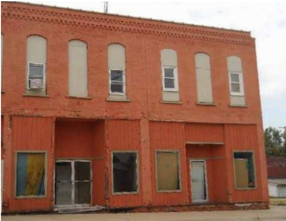
Filling in existing window openings with smaller windows, as seen here in a building in Illinois, is not recommended in Laurel.
