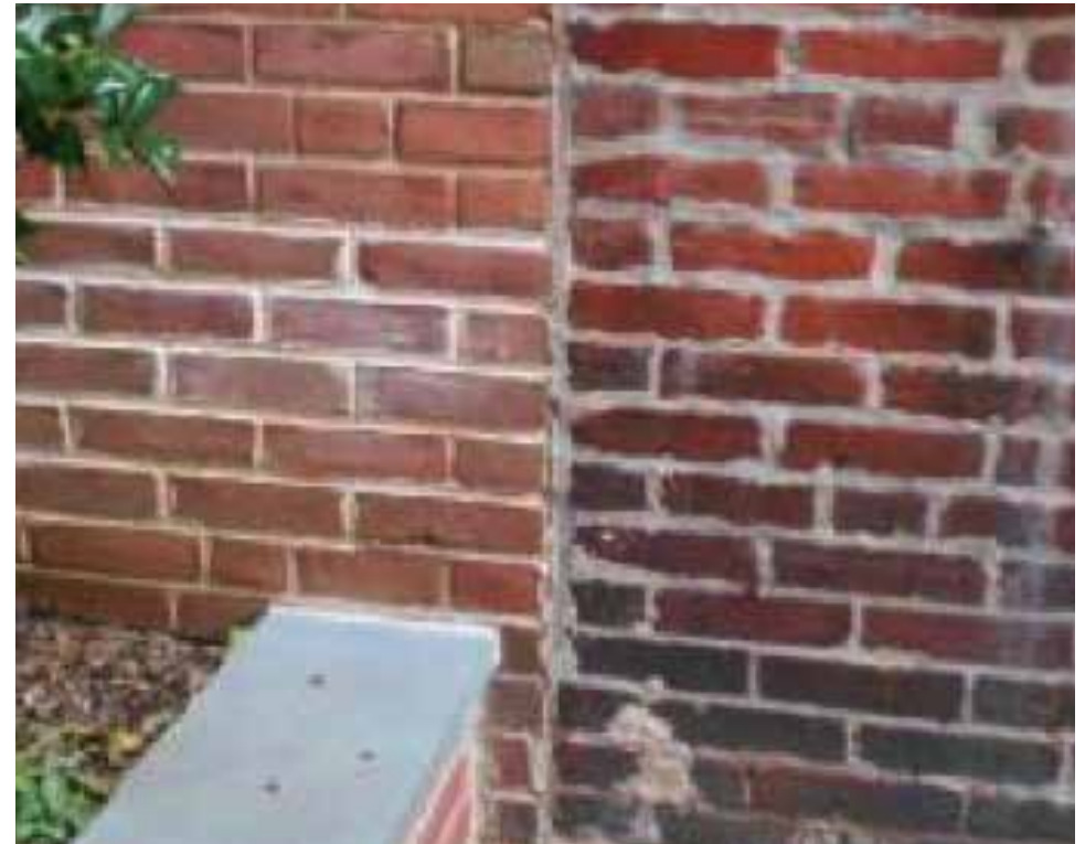
The pointing in the upper left-hand portion of this brick building in Philadelphia has been pointed correctly, while the brick pointed on the right side has been poorly applied. The right side shows where the new mortar has been permitted to “feather edge” onto the face of the adjacent bricks, which is not recommended.
