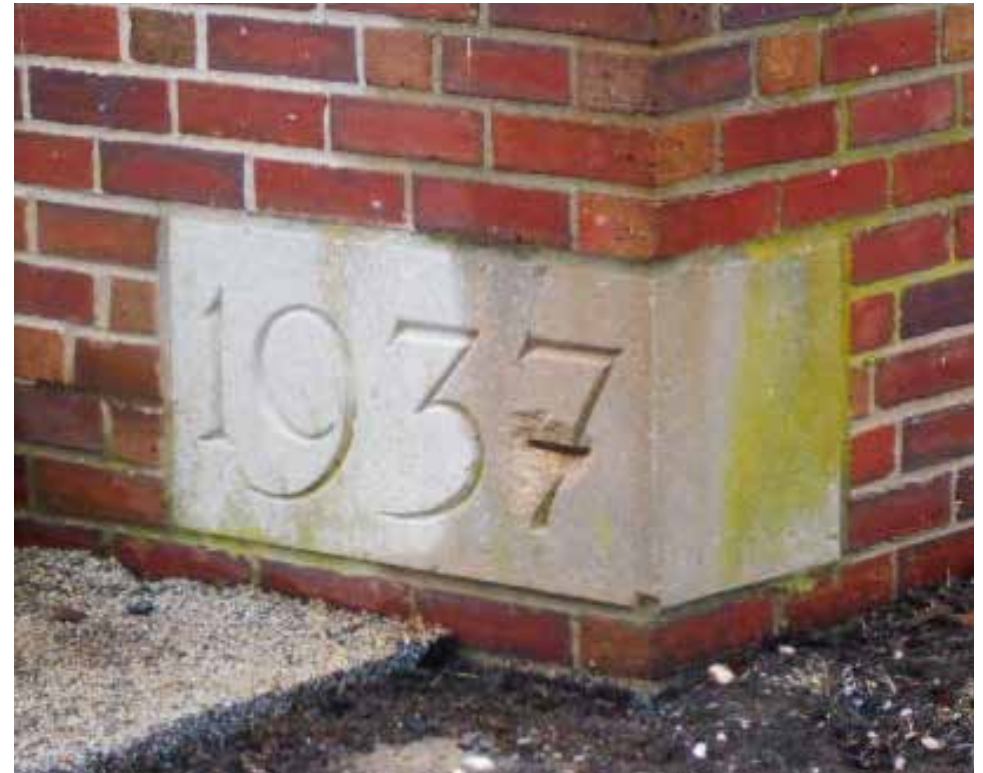
When repointing, match the width and profile of existing mortar joints, as seen here on Town Hall at 201 Mechanic Street. Use the same tooling pattern as the original joints. Your contractor should match the color and texture of the new mortar to the existing mortar. Mortar gets its color from the sand used, so choose sand that is comparable in color and texture to the grain used in the original mortar when repointing.
