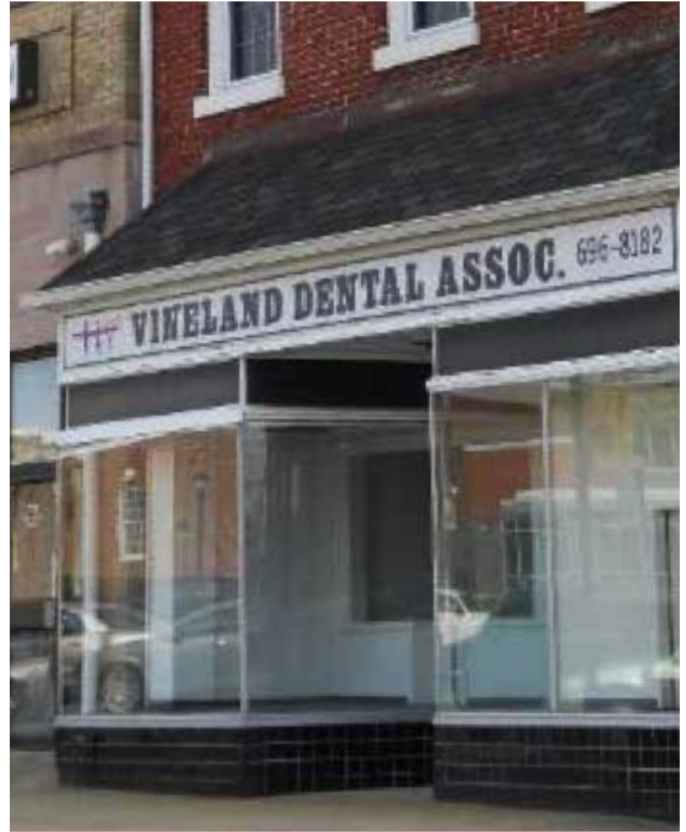
Keeping storefront display windows empty is not recommended as seen here on a building in Vineland, NJ.
