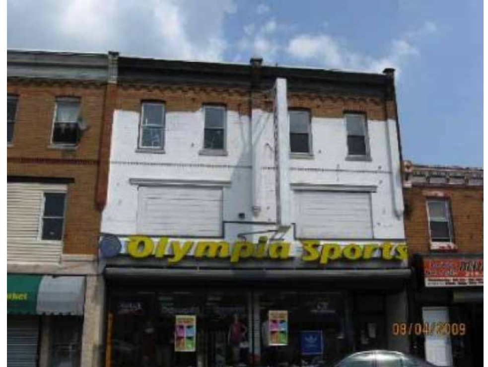
It is not recommended to paint brick (see above), stone, tile, stucco, or molded concrete block if they have never been painted before, as seen on this building from Philadelphia. The unpainted elements have a natural or man-made exterior finish that is important to preserve.
