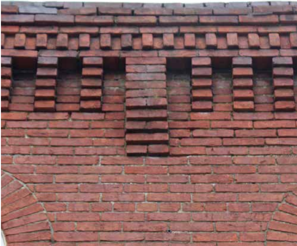
The brick cornice at 122 East Market Street is original to the building and should be retained.
