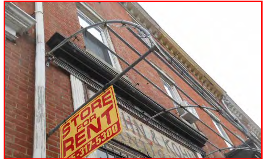
Avoid retaining metal armature of an awning attached to a building without its canvas covering.
