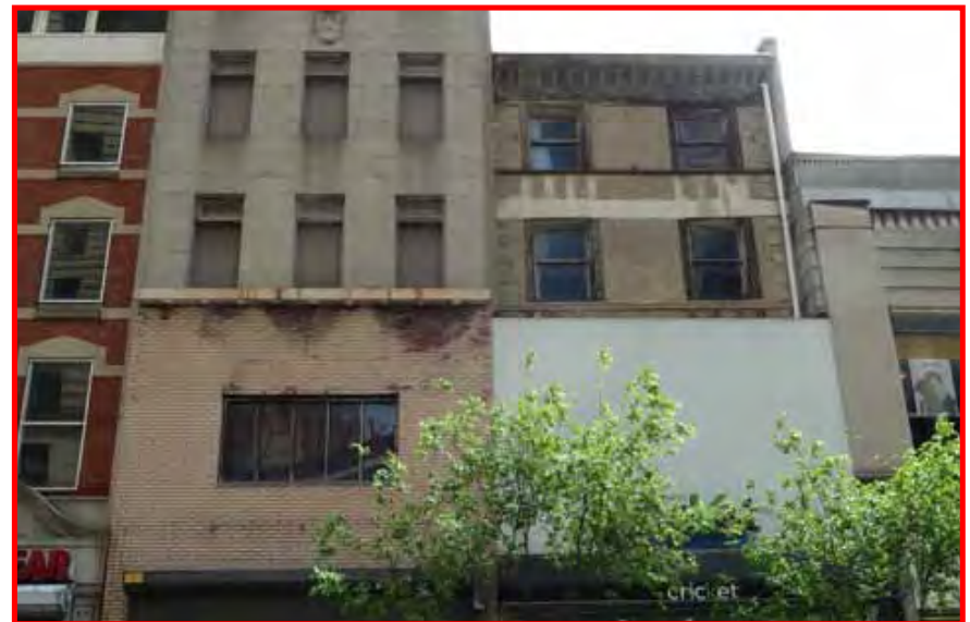
Avoid creating windowless, blank walls by destroying or covering original architectural details.
